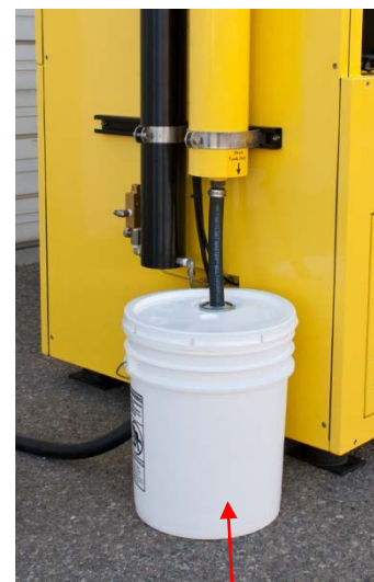
Condensate Drain Container Check & Drain Daily
